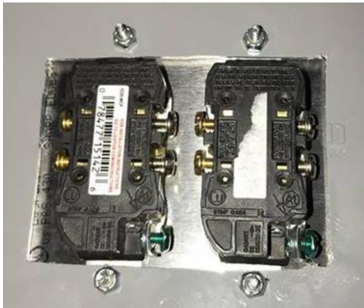
Figure 3-6 – Outlets mounted to stainless-steel cover and lid enclosure
